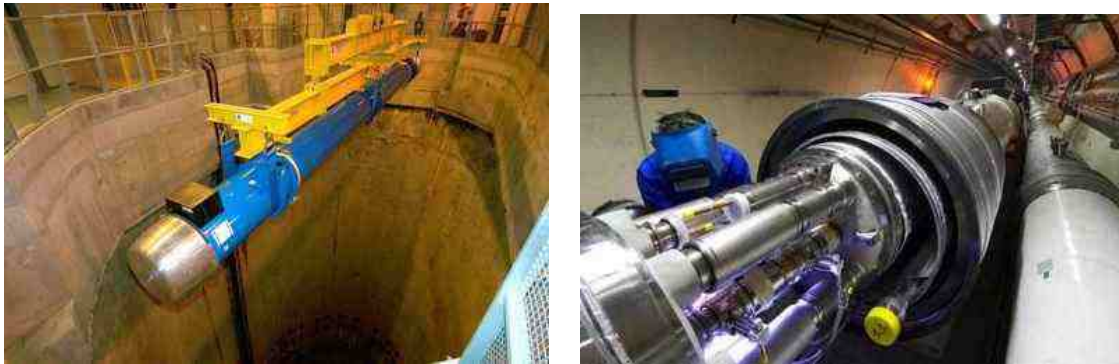
Figure 1: Left : Lowering of the first superconducting LHC dipole into the tunnel, March 2005. Right : Interconnection of two dipoles, next to the cryogenic services line.
