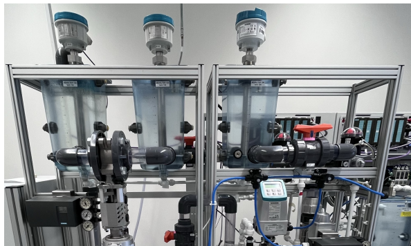
Fig. 3. Three tank hardware test bed at the model factory of Institute of Automatic Control, RWTH Aachen University .
