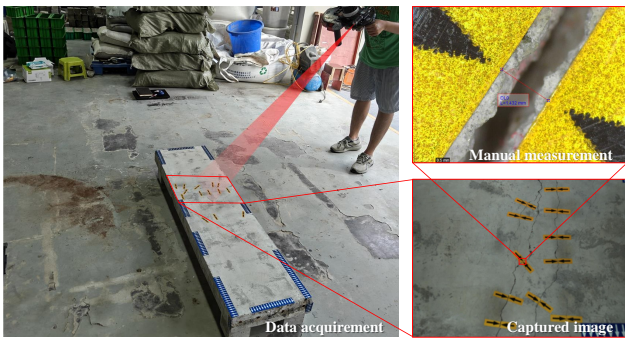
FIGURE 14 Field Operation for Concrete Slab: This figure illustrates the data collection process for the concrete slab, along with the corresponding data. It also shows the measurement of crack true values using a Dino-Lite AF4915 microscope.
