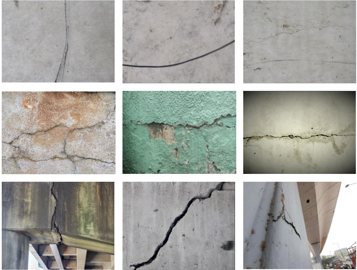
Figure 2. Example of concrete crack images considered in the dataset
