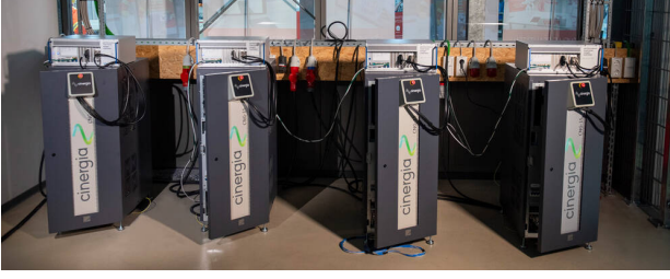
Fig. 4: Four inverters in the power hardware in the loop lab. While structurally similar, the implemented control differs significantly from the EMT model.
