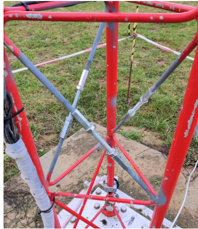
FIGURE 13. Photograph of reversible damage mechanisms integrated into the struts of the girder mast structure.
