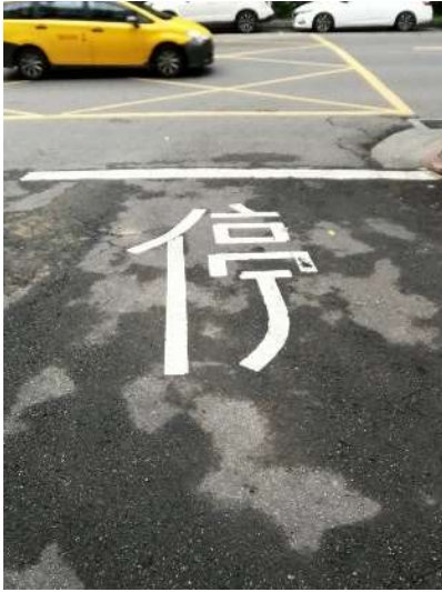
(a) Stop sign – Lane 92, Sec. 2, Xiuming Rd.
