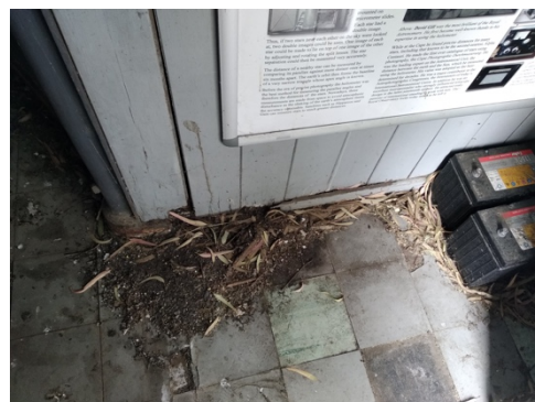
Figs 18 & 19: The interior of the building, showing the result of bird invasion and leaks.
