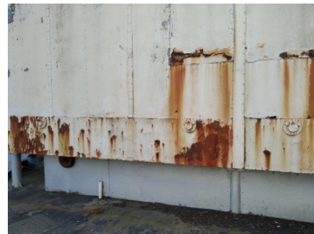
Fig 17: Typical examples of rust on the outside of the building.
