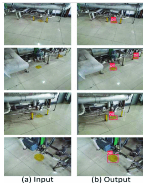
Fig. 3: Detection of oil leakage based on CBAM-YOLO v5.
