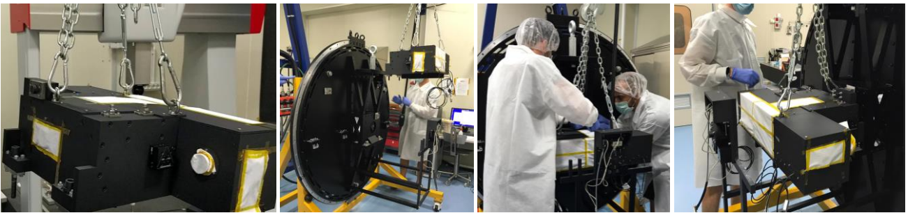
Figure 25. From left to right: CP lifted; CP in front of the IF flange; tightening of the CP KMs; CP installed.
