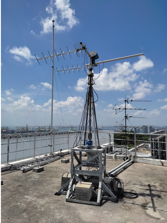
Figure 3: Singapore UHF ground station on the roof top at NUS campus.
