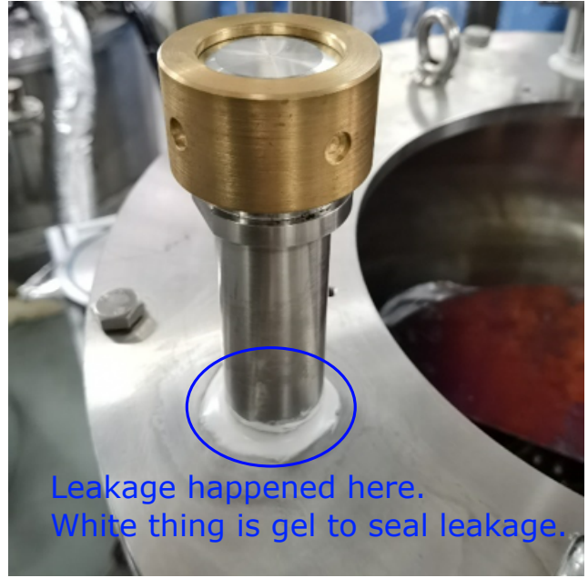
Fig. 15b. The welding place of the LHe inlet on the vacuum vessel had a leakage. Vacuum gel was used to seal the leakage successfully.
