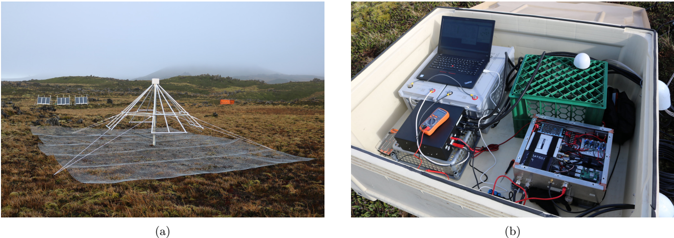
Fig. 5: (a) Single autonomous station pathfinder installed at the hydro shack site. The system is powered by a bank of solar panels that are visible in the background. (b) A weather-proof container, which sits near the solar panels, houses the batteries, solar charge controller, and readout electronics.
