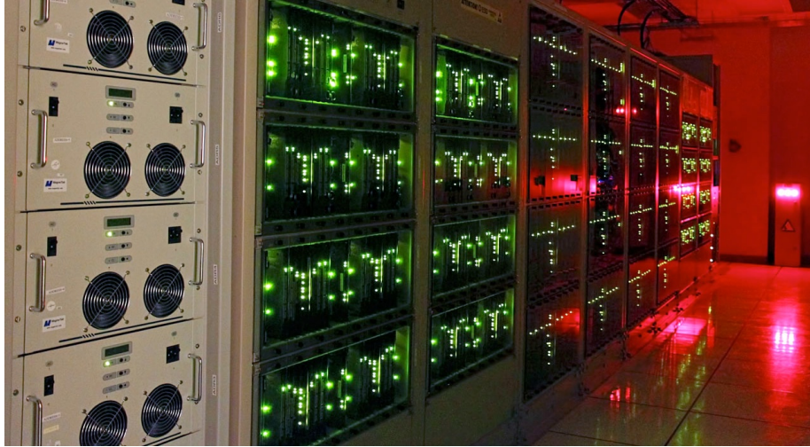
Figure 4: One quadrant of the ASIC-powered ALMA correlator. The ALMA correlator processes up to 16 GHz bandwidth from 64 antennas. Image credit: ALMA (ESO/NAOJ/NRAO), S. Argandoña
