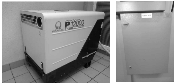
Fig. 2. Generator ProTech P12000 and ATG system
