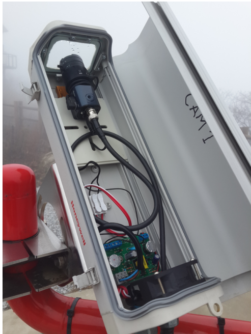
Figure 5. Detailed view of the interior of the protective camera housing of SOAO camera 1. Both the coaxial video-signal and 12V camera power cable (white/red) are visible. Additional electronics controls the housing fan (mounted on the rear-end and heater (placed under the camera lens beneath the housing front glass). See online version for colors.
