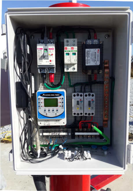
Figure 7. Detailed view of the power supply (main switch) box with automatic operation (Dong Hwa) timer (at SOAO). Black boxes on the top-left side are the three 12V power supply transformers for the Watec cameras. See online version for colors.
