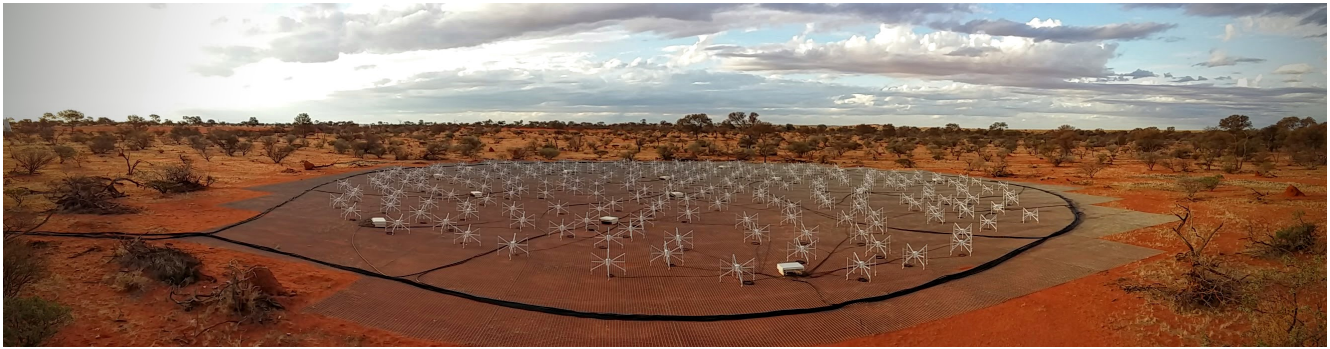
Figure 4.: A panorama of the EDA looking north. In-field beamformers (small white boxes) each service 16 dipole antennas. The thick black cables are the 200 m coaxial cables running between the beamformers and the shielded room.
