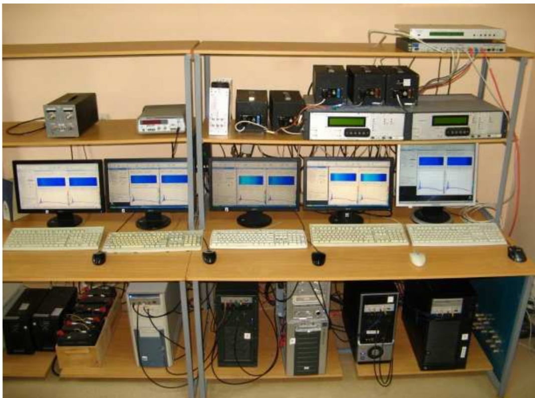
Fig. 5. The set of five DSPZ (one per telescope beam) installed in the UTR-2 receivers room.
