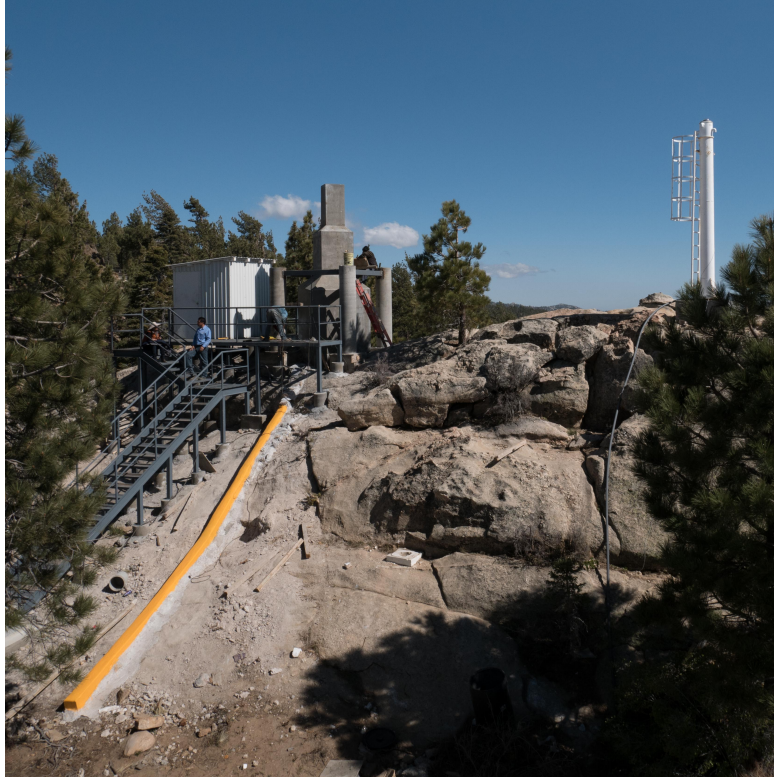
Figure 5. The COATLI installations at SPM. The ARTS platform will be mounted on the four smaller columns (three of which are visible). The telescope and mount will be mounted on the massive central column. The shed to the left will contain the control computers and electronics. The installation is on a rocky outcrop to the south east of the existing 84-cm telescope. The white mast is an existing all-sky camera.
