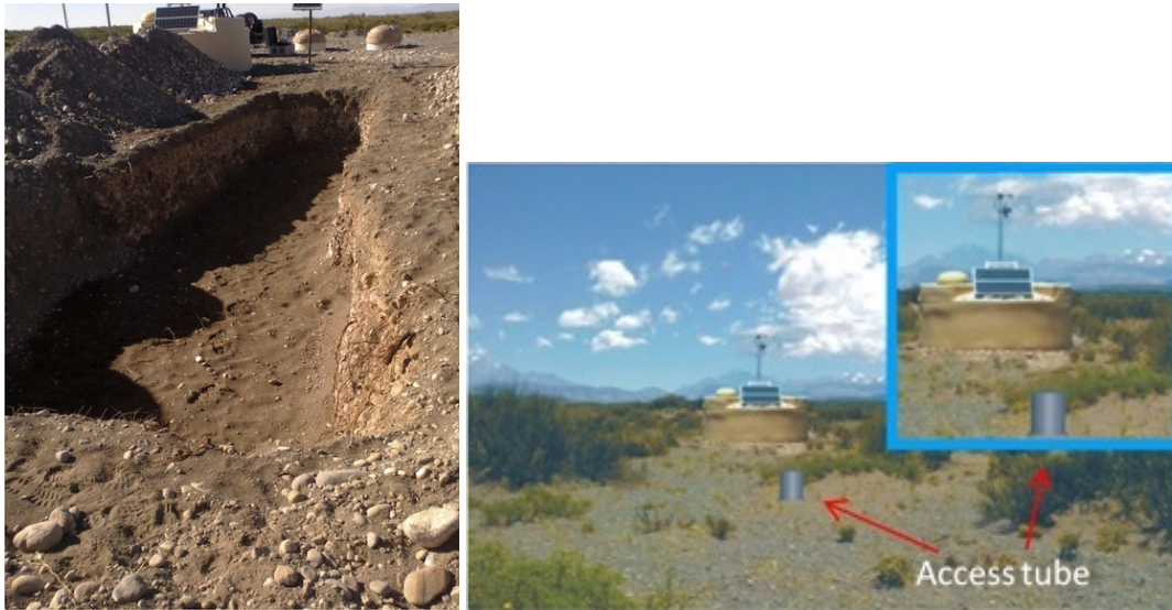
Figure 9.3: Left: 1.3 m deep hole for a 10 m 2 module; Right: photograph of final deployment.
