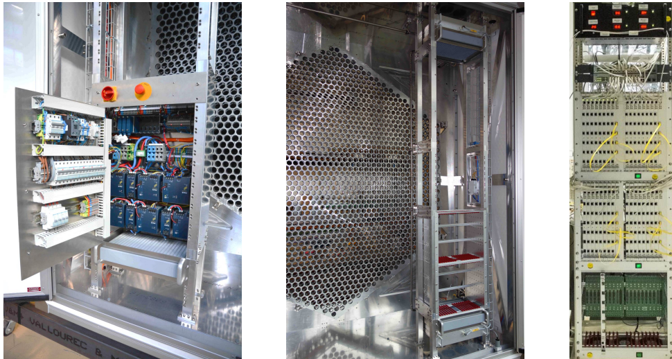
Figure 4: Photos of the FlashCam prototype camera. Left: Safety control cabinet installed inside the camera body. Middle: rear view into the camera body showing one of the installed electronics racks and an attached cooling pipe. Right: Rack with readout electronics under test.
