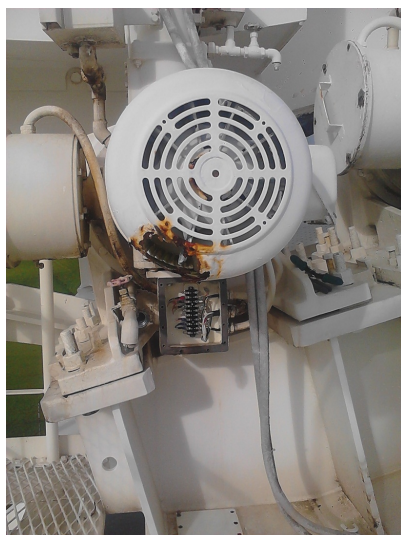
Figure 5. The state of the old motors was very poor and was considered a safety issue. (Image courtesy of Stuart Weston)
