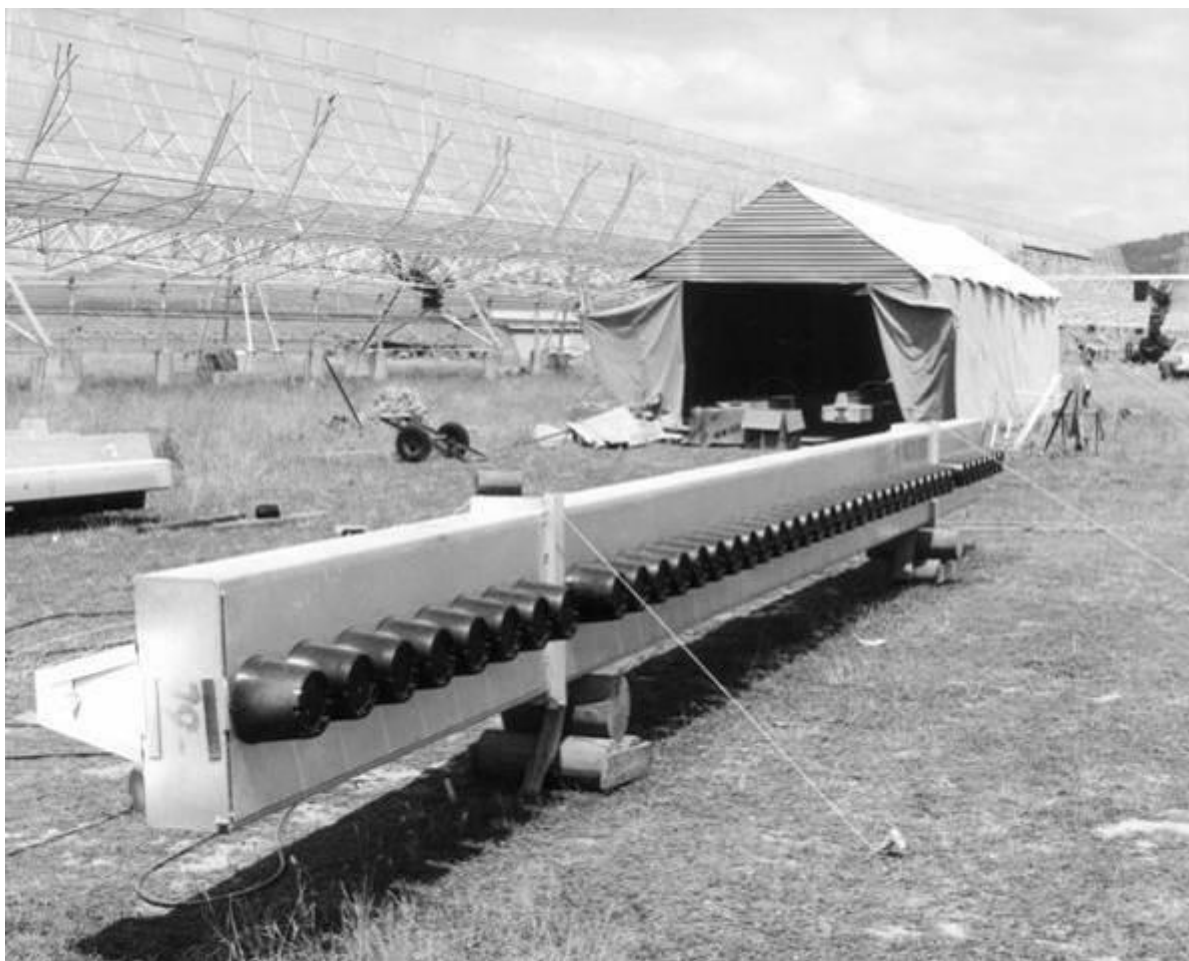
Figure 10: The construction of MOST showing the new feed elements designed to operate at 843 MHz. In the MOST configuration only the east-west arm (visible in the background) of the original cross was used (courtesy of the University of Sydney Archives).
