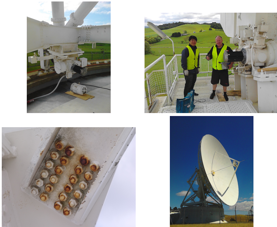
Figure 2: The 30m, Top-left one of the old azimuth motors being replaced. Top-right Tim and Takiguchi having finished replacing one of the elevation motors. Bottom-left an example of the corrosion we have to get on top off. Bottom-right with the new motors and control system we are now able to move the dish once again. Image Credit: S. Weston
