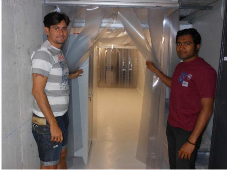
Figure 6. A view of the entrance in the clean-room already installed in the LARIX tunnel.
