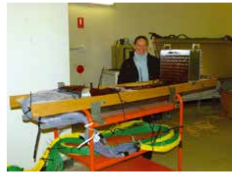
Figure 6. Kristin Fiegert (fibre optician) with the HERMES and AAOmega fibre optic cables, ready to be inserted into the conduit.
