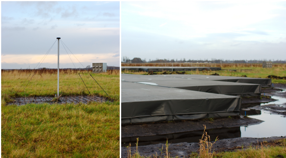
Fig. 1: Antenna types of the Low-Frequency Array. Left image: A low-band antenna with a cabin in the background. Right image: Part of a high-band antenna station, consisting of 24 tiles of 4 \times 4 high-band antennas.
