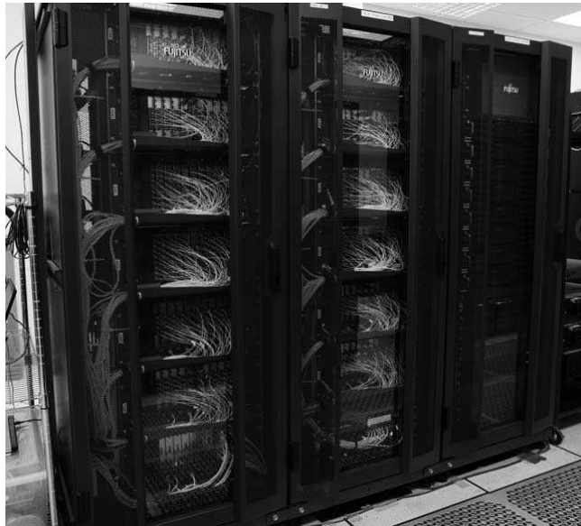
Fig. 9. A quadrant of the ACA Correlator. The left and middle racks compose a quadrant, which processes a baseband pair from sixteen antennas. The right rack is one of four computing racks, which have correlator control, post processing computers, network instruments and so on.
