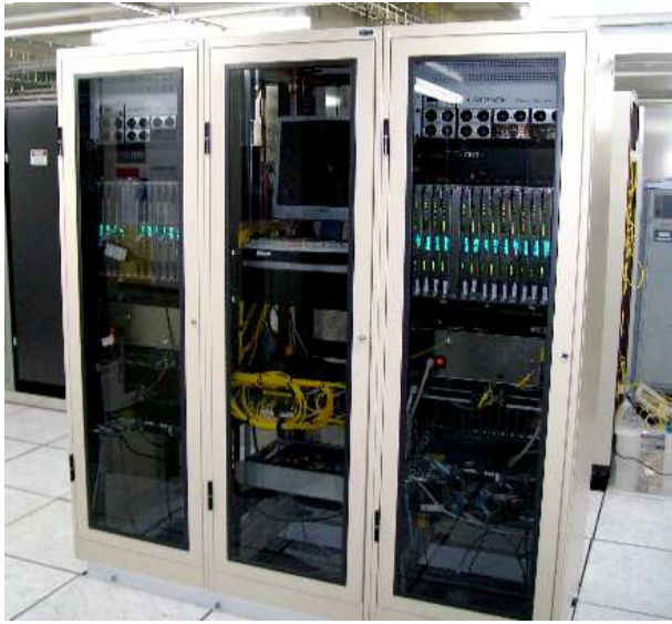
Figure 14. The CABB rack as installed in the fully shielded ATCA correlator room.
