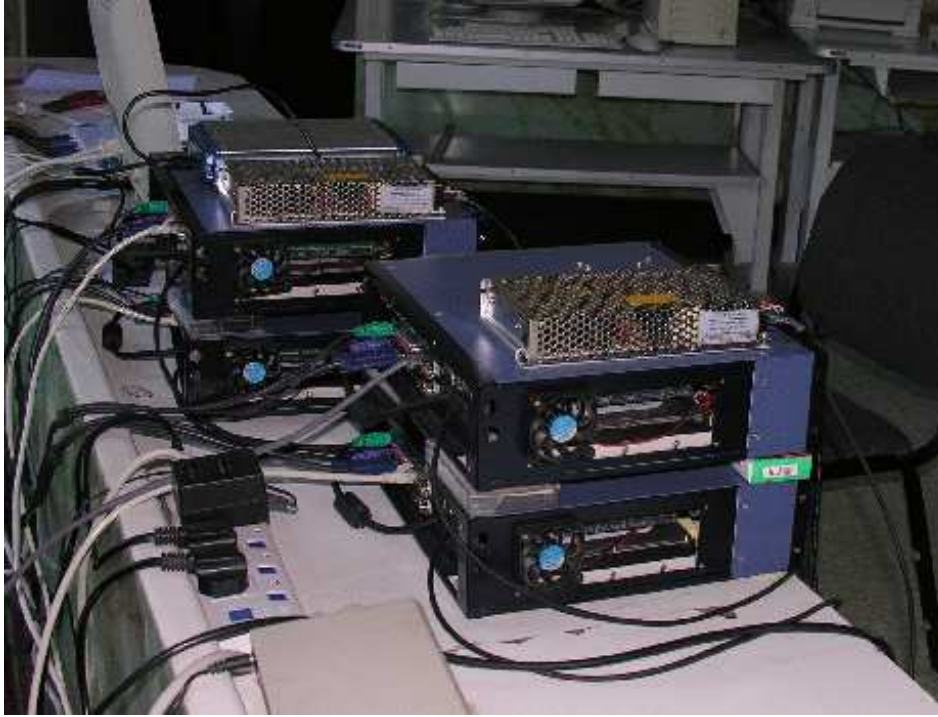
Fig. 5 Computer control equipment.
