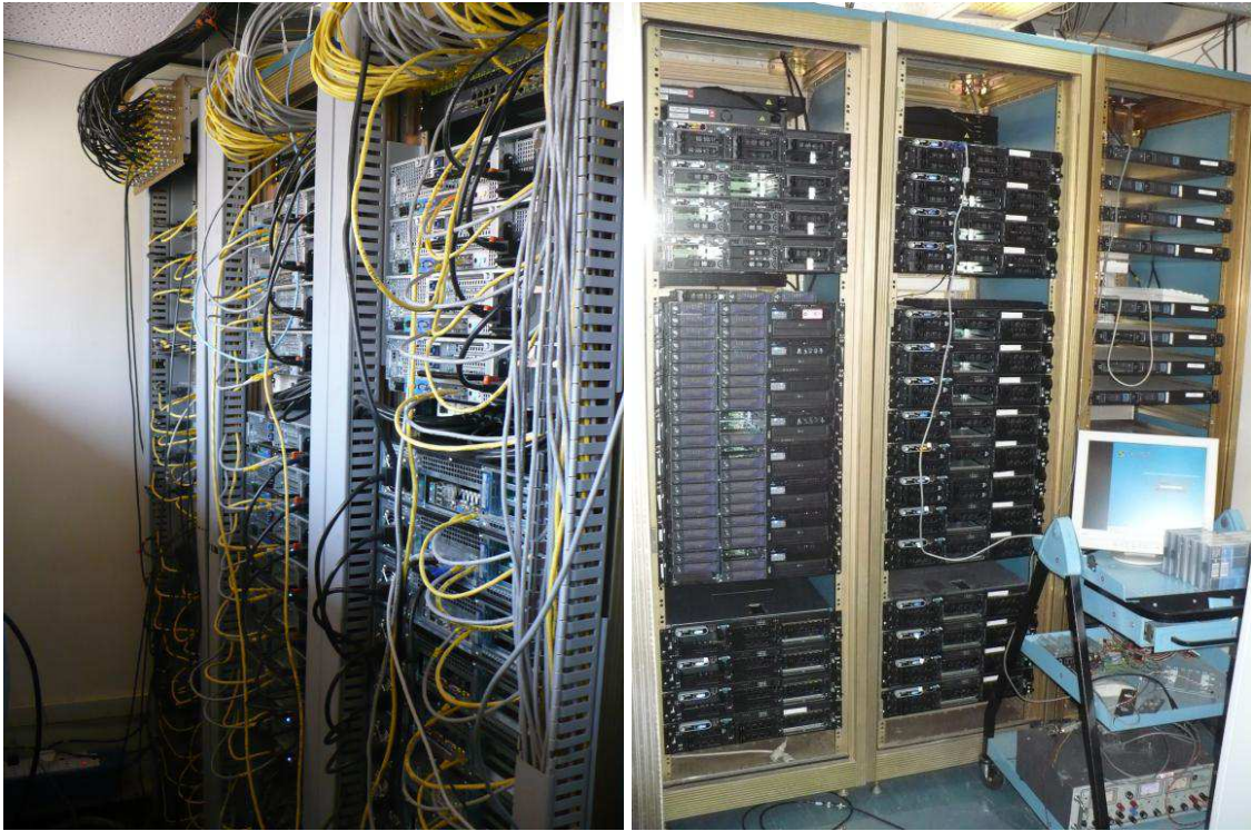
FIGURE 4. The newly installed GMRT software back end. It allows a wide variety of modes, including software correlation, and recording of all raw voltages to disk.
