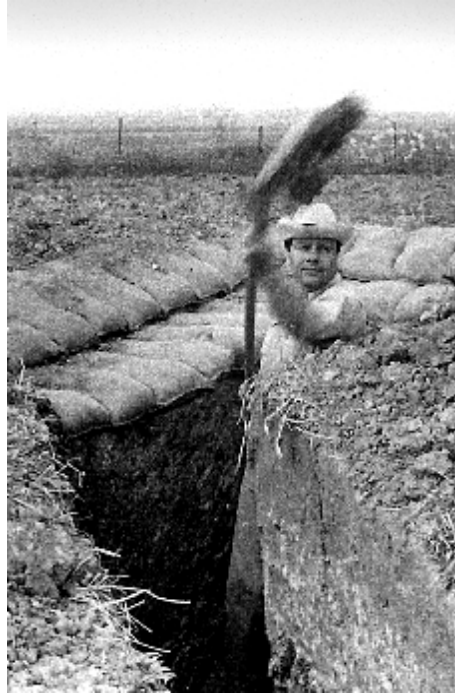
Fig. 5 Racah digging trenches in Kibbutz Deganya Alef during Operation Bitzurim, when all classes at the Hebrew University were suspended for a week to enable teachers and students to assist in the work of building fortifications in the border settlements (29 April – 4 May 1956) [Courtesy of Dr. Eli Racah].
