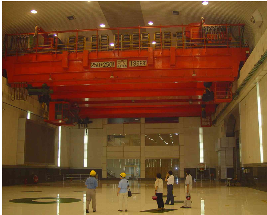
Fig. 4.12. A photo of a bridge style crane, the crane rail is fixed to the wall of the experimental hall.
