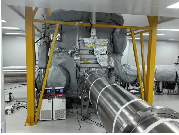
(a) Central tank featured in the lab, which has a lift that can be lifted up by the crane. It is 3.5 meters tall and 2.5 meters in diameter.
