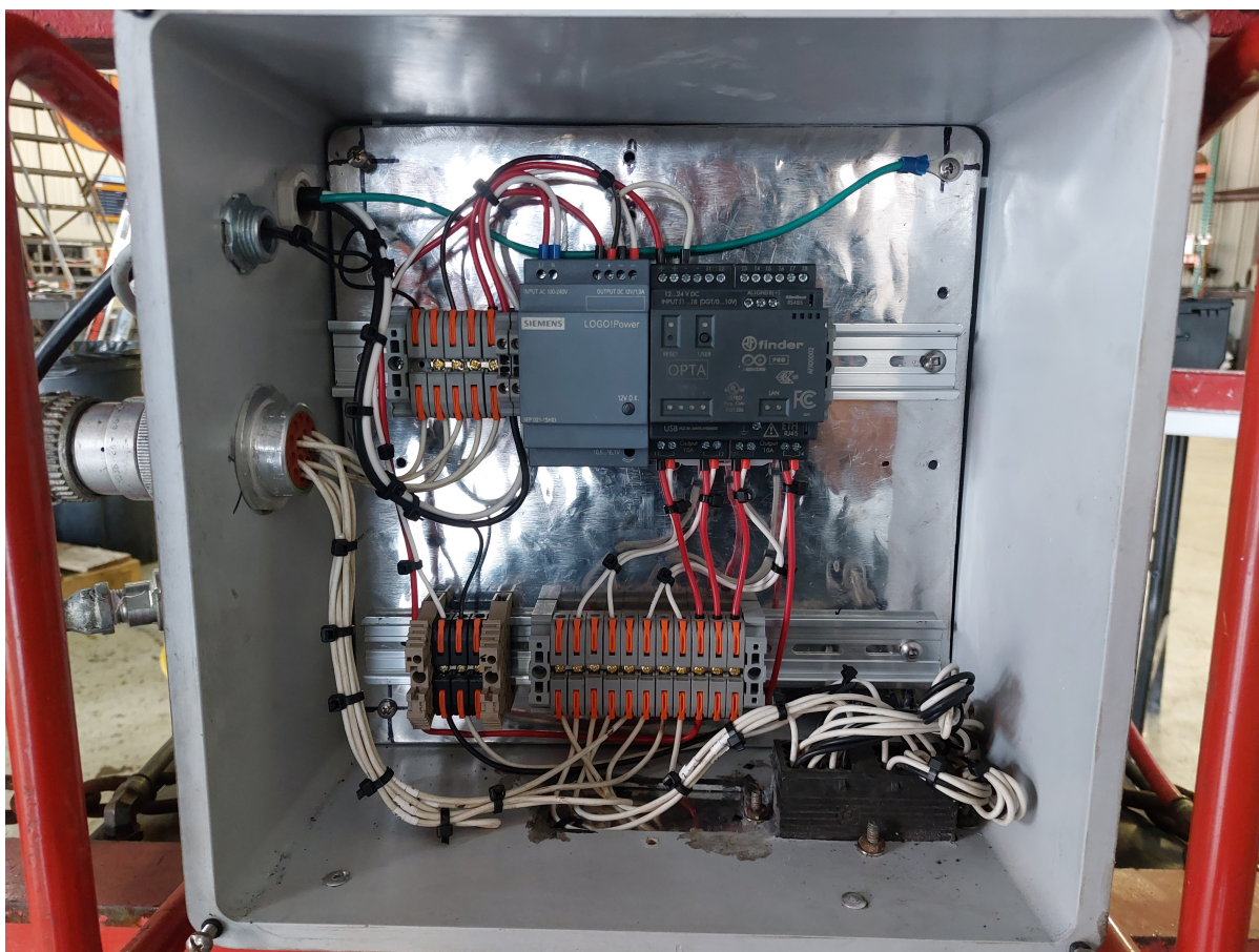
Figure 5: Assembly of the automatic control prototype designed for the automation and monitoring of the cyclone.
