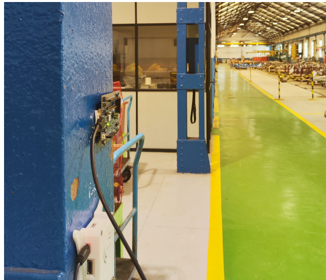
Figure 19. Transmitting node in the workshop.
