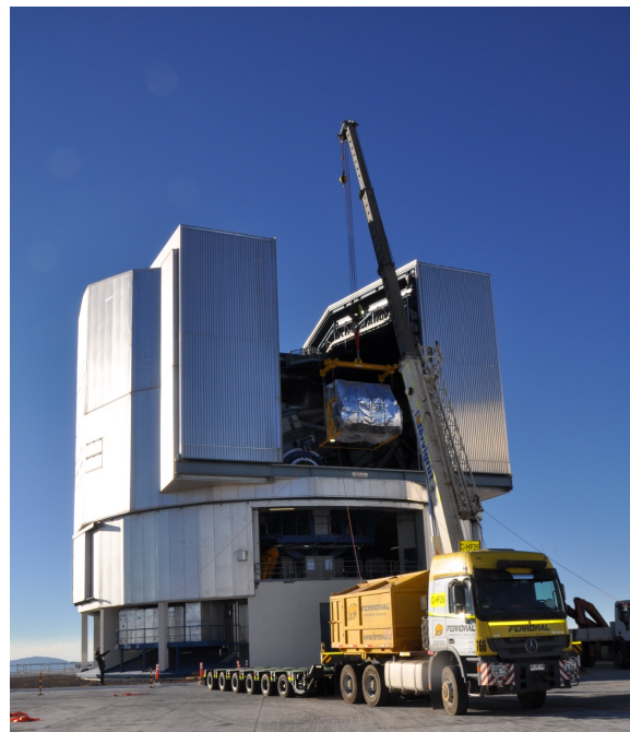
Figure 9: MUSE "landed" on the UT4 Nasmyth platform on January 19, 2014.
