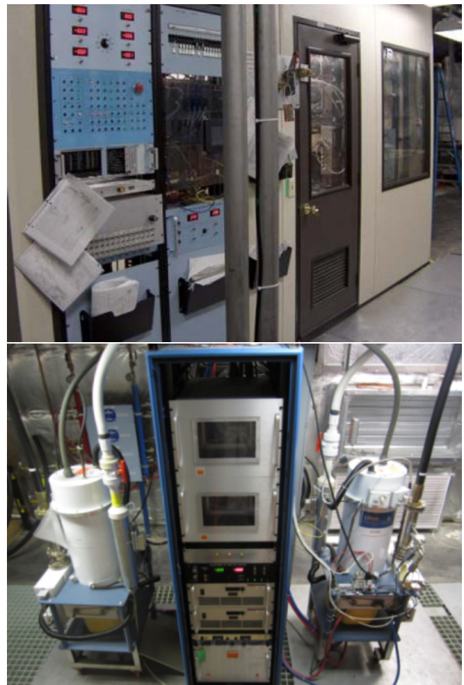
FIG. 36. The 20 kV High Voltage enclosure and controls above and a pair of 10 kW IOTs with their controls below.
