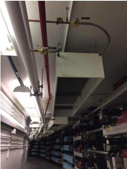
FIG. 48. Photograph of chilled beams of the air conditioning system next to the East Arc magnets
