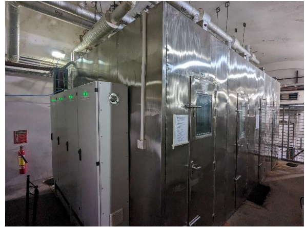
Figure 4: Practical Implementation of the Stability Chambers
