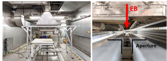
Fig. 3 Aperture slit setup with oscillating irradiation box below ELV-2 (left). Close-up of electron exit window with an adjustable aperture below (right).
