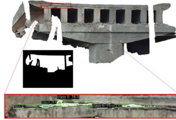
(e) Bridge Capture and Crack Detection
