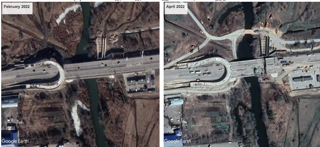
(d) B17: LoK H ; DL M ; CCD GL =0.351; CCD LOC =0.521 (on the right a temporary diversion route was constructed to bypass the bridge)
