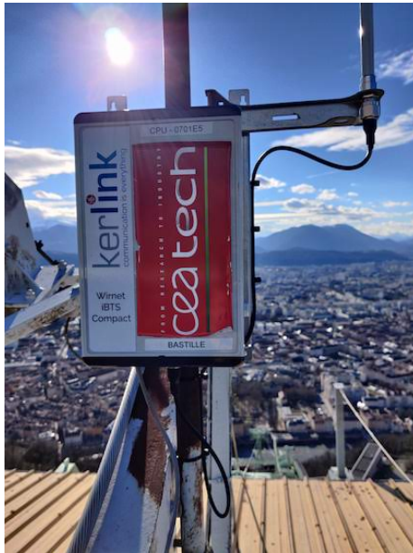
Figure 8: Gateway BS_3 which is installed on the roof near the cable car station at Bastille, Grenoble
