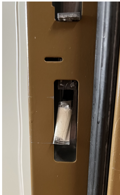
Figure 6.3: Door lock sensor.
