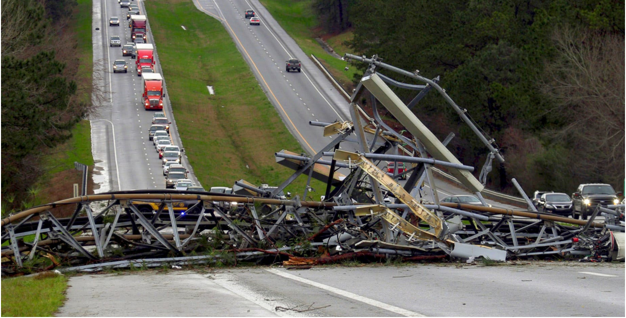
Fig. 1. Disaster-struck cell tower [14].
