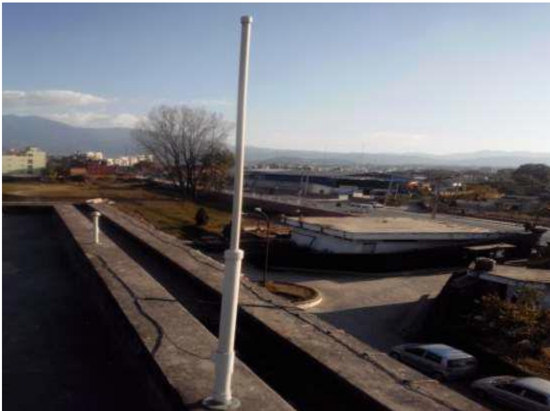
Figure 2.2: Photograph of stroke antenna and GPS antenna on rooftop of NAST.
