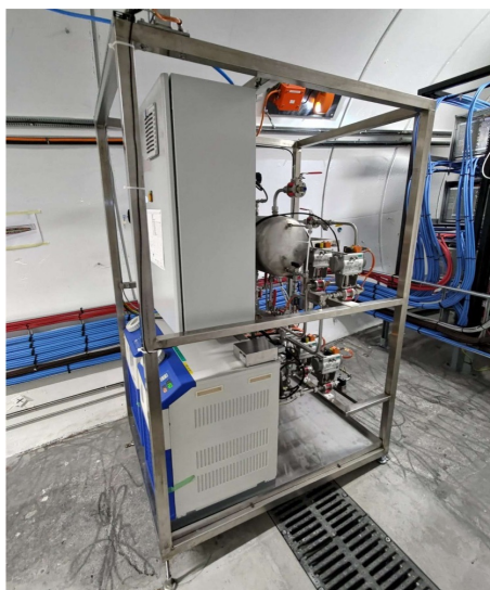
Figure 16: Photograph of the cooling system.
