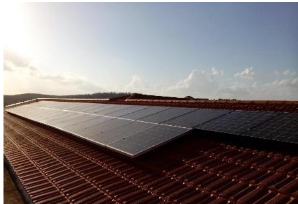
Figure 1 - Rooftop PV system with 6740 W installed power, in one of the UÉvora's microgrids.
