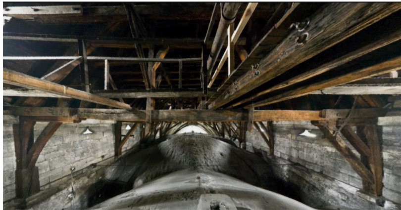
Figure 5: The charpente of the choir; the top of the guttering wall was, before \sim 1220 , at the level of the corbels supporting the wall pieces and braces beneath the fermes .
