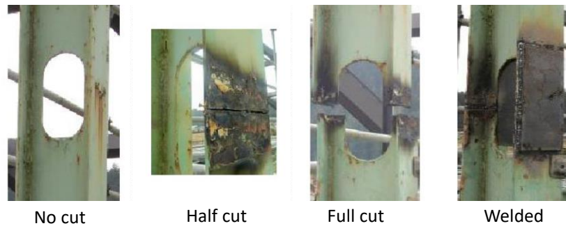
Figure 16 – Damage cases on the flanges of vertical truss member at the bridge midspan in Goi and Kim [135].
