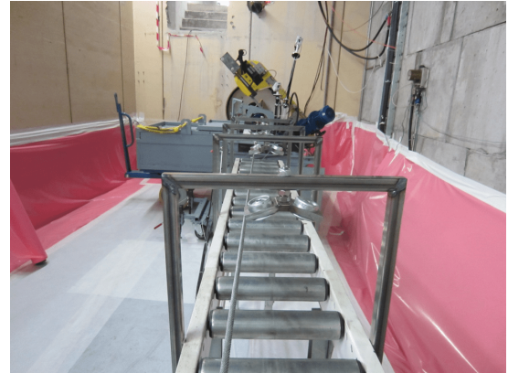
FIG. 17: Tooling for the extraction of the original dump core and beam pipe out of the dump cavity. In the foreground, the support structure with rollers and the winch cable. In the background, the remotely operated saw and the lead-shielded container.
